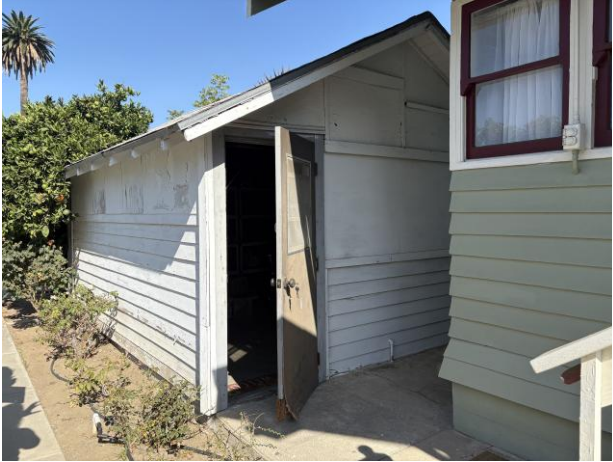
Figure 14. East façade (foreground) and south façade (left) of ancillary building, view northwest
