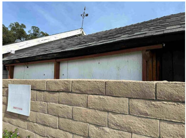
Figure 10. The north end of the garage's rear (west) façade of the garage, which is enclosed under the roof eave, view northeast. Source: DSEA, Inc., January 2026.
