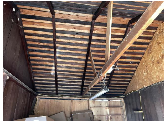
Figure 12. Interior of the north garage bay, view west. Non-original wood cladding seen at the west (center) and north walls (right)
