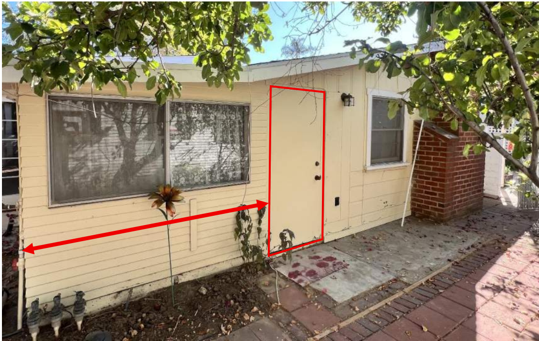
Figure 29: View of existing north [side] façade with area to be demolished/alterd to accommodate proposed bedroom addition. An existing slab style door will also be replaced. Source: JANUS.
