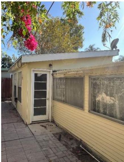
Figure 37: View of existing exterior rough sawn plywood cladding and windows to be replaced at rear bedroom [facing south]. Source: JANUS.
