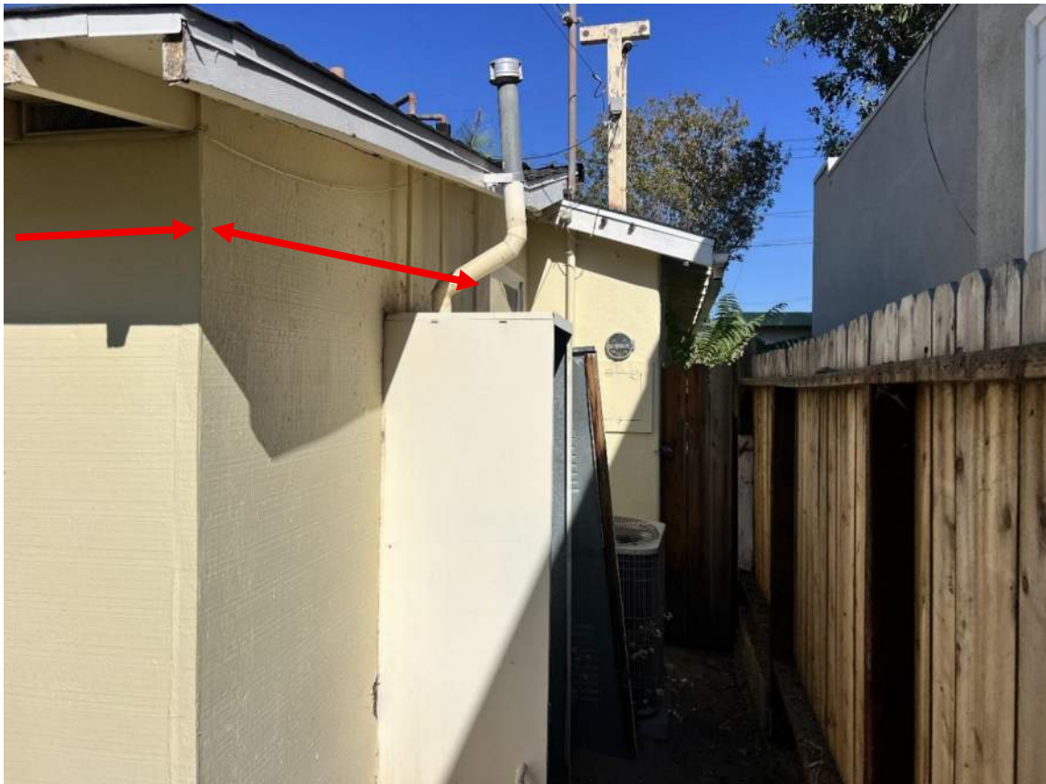
Figure 23: View of existing primary bathroom [to be demolished] with exterior water heater cabinet [facing east]. Source: JANUS
