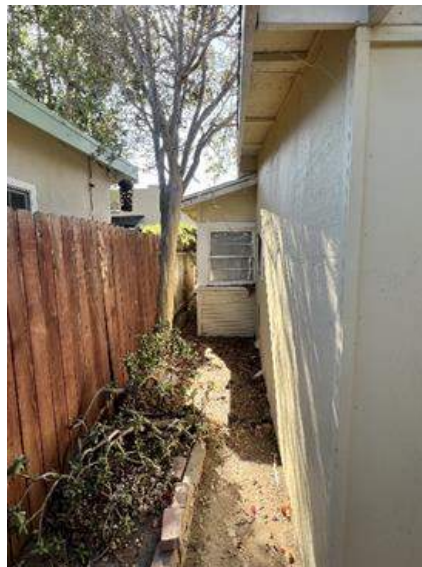
Figure 38: View of existing exterior rough sawn plywood cladding and windows to be replaced at rear bedroom [facing west]. Source: JANUS.
