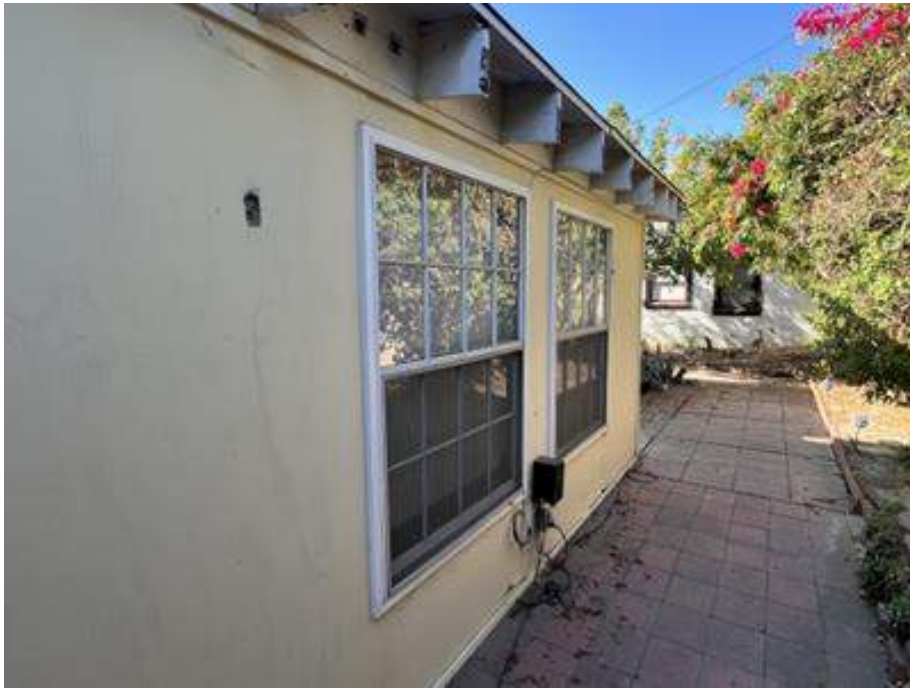
Figure 36: View of existing exterior rough sawn plywood cladding and windows to be replaced at rear bedroom [facing north]. Source: JANUS.
