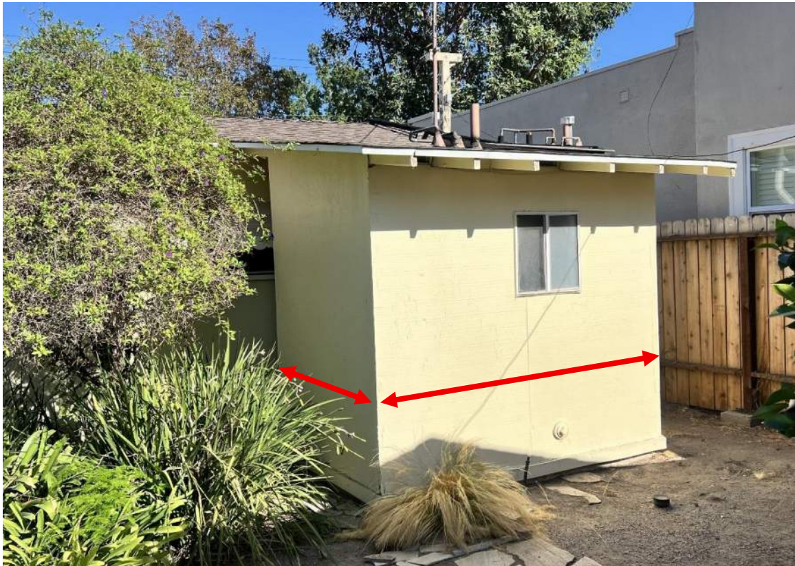
Figure 22: View of existing primary bathroom [to be demolished] with rough-sawn plywood siding and aluminum sash window [facing southeast]. Source: JANUS
