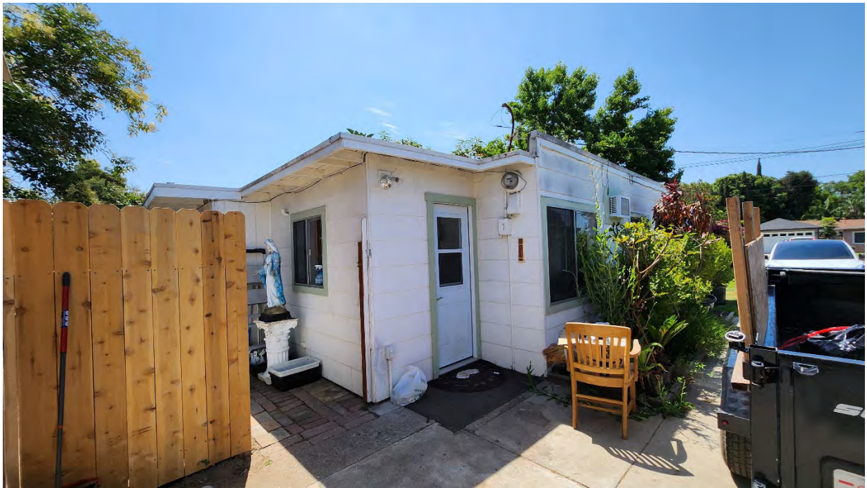
Figure 10: North (left) and west (right) elevations, view facing southeast. Source: GPA Consulting, July 2024.
