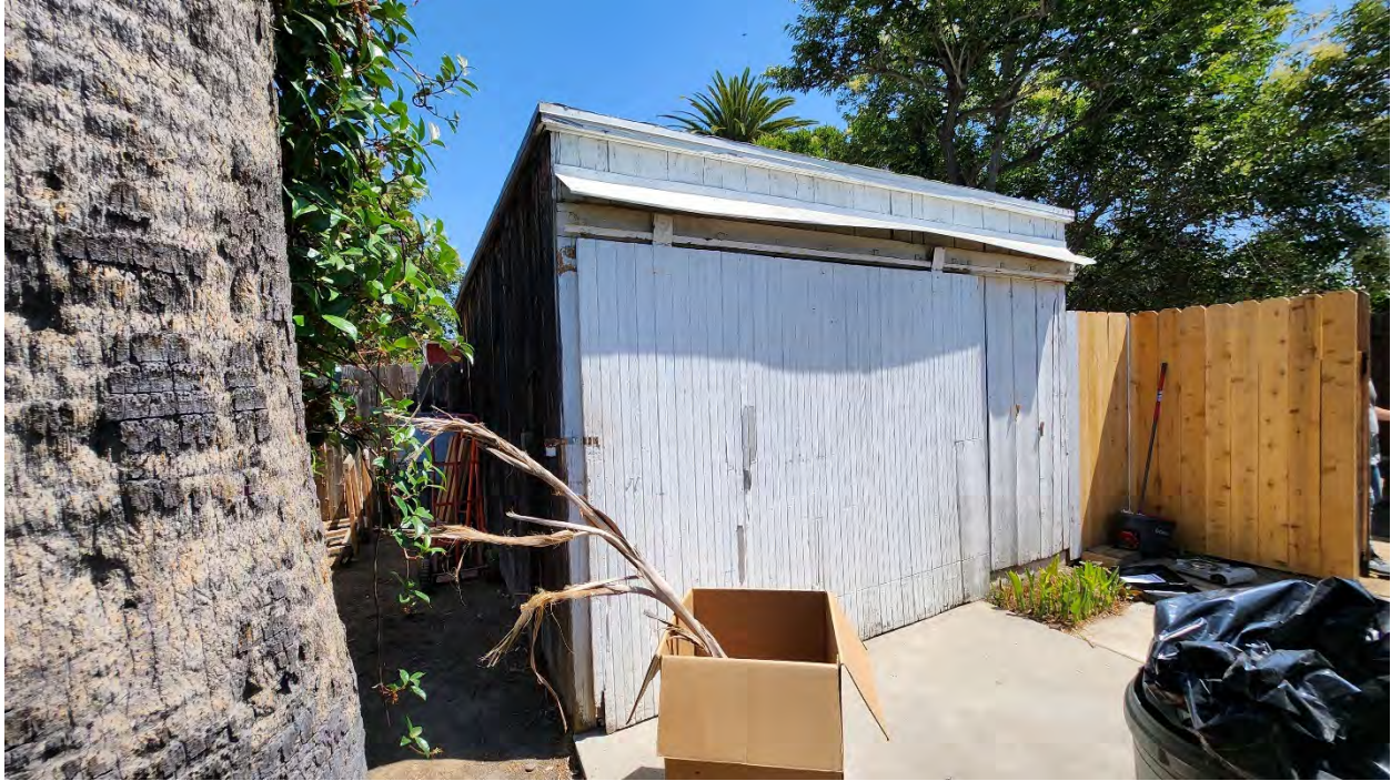
Figure 13: West (left) and south (right) elevation of garage, view facing northeast. Source: GPA Consulting, July 2024.
